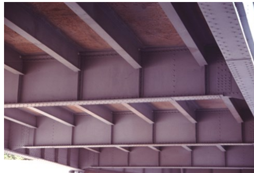
Bridge coated with WB HRZS Single Coat System, after 17 yrs. in service.
