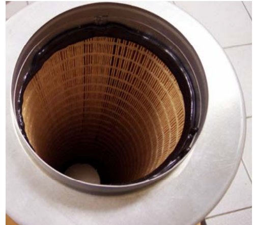
Filter sealed with Rigid Foam Adhesive
